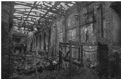
FIG. 2. An illustration of some of the damage caused by the fire in St. George's Hall.
