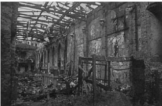
FIG. 2. An illustration of some of the damage caused by the fire in St. George's Hall.
